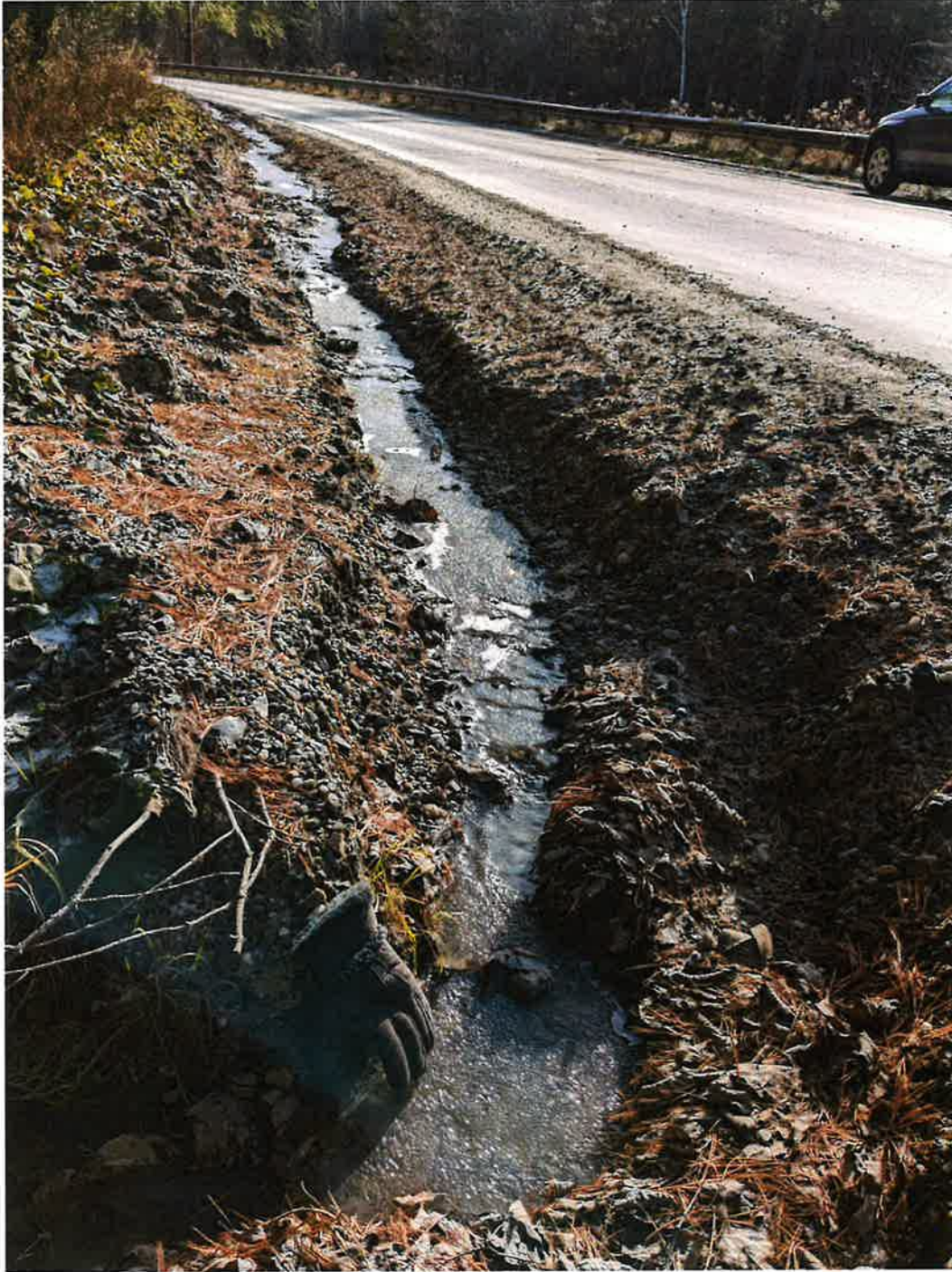
Grader ditch on north side of Nashville Road that will be excavated and stone lined. Notice glove in foreground for scale.
