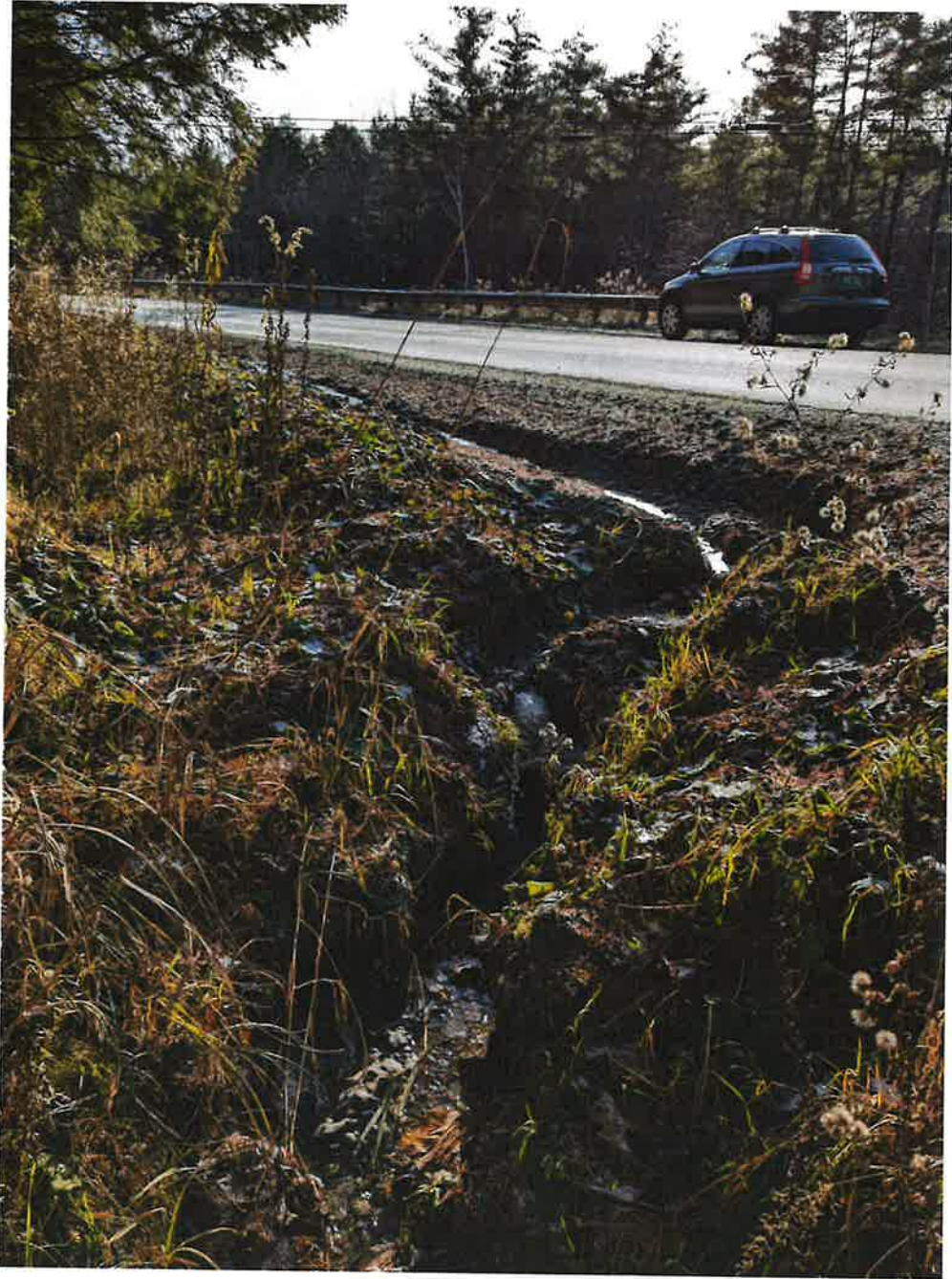
Erosion in existing ditch line on north side of Nashville Road. Note grader berm that will be removed as part of this project.
